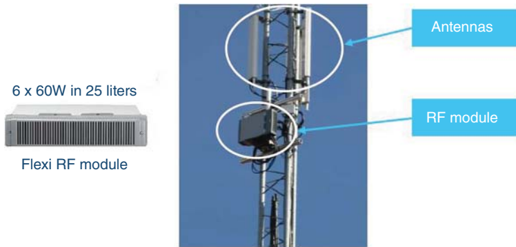
Figure 14.8 Compact Nokia RF module site solutions [9].
